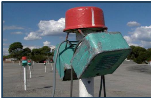
The distinctive speakers and junction boxes installed were used only by Wallis.
