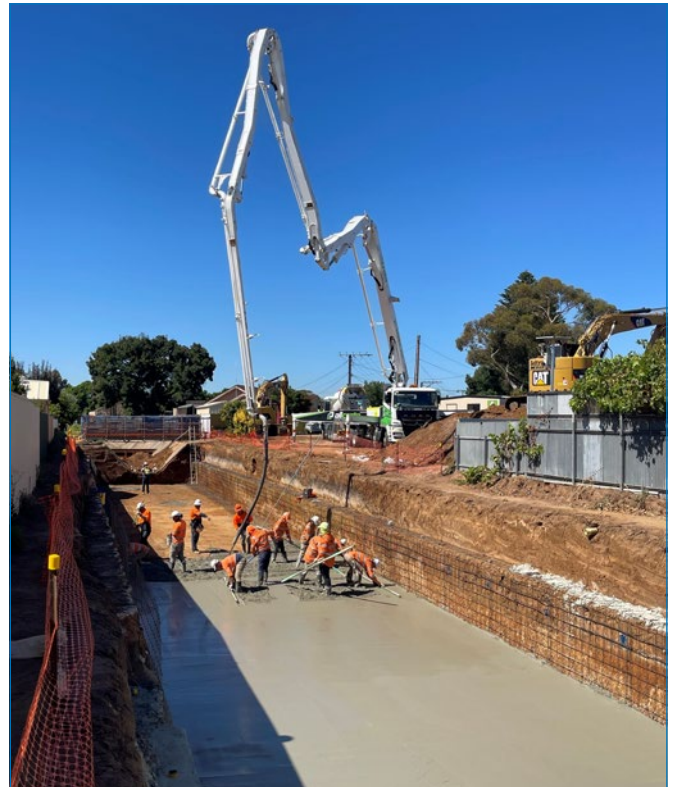
The protective concrete layer being installed on the floor of the channel excavation.
